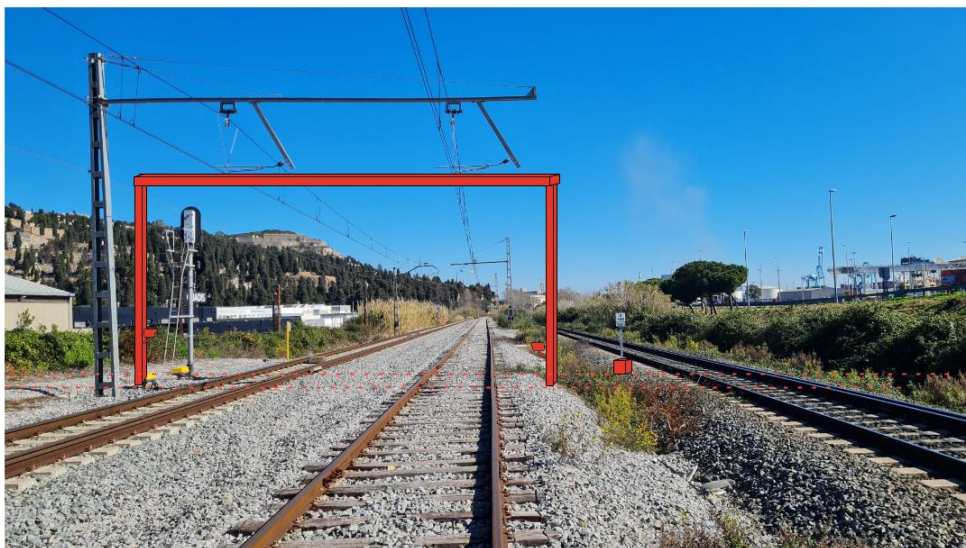
Figure 7.40 Checkpoint for double-track railway installation at Morrot location.
