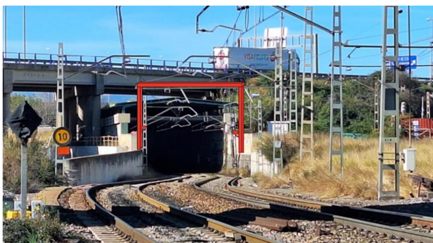
Figure 7.42 Checkpoint for double track railway installation at Llobregat location.
