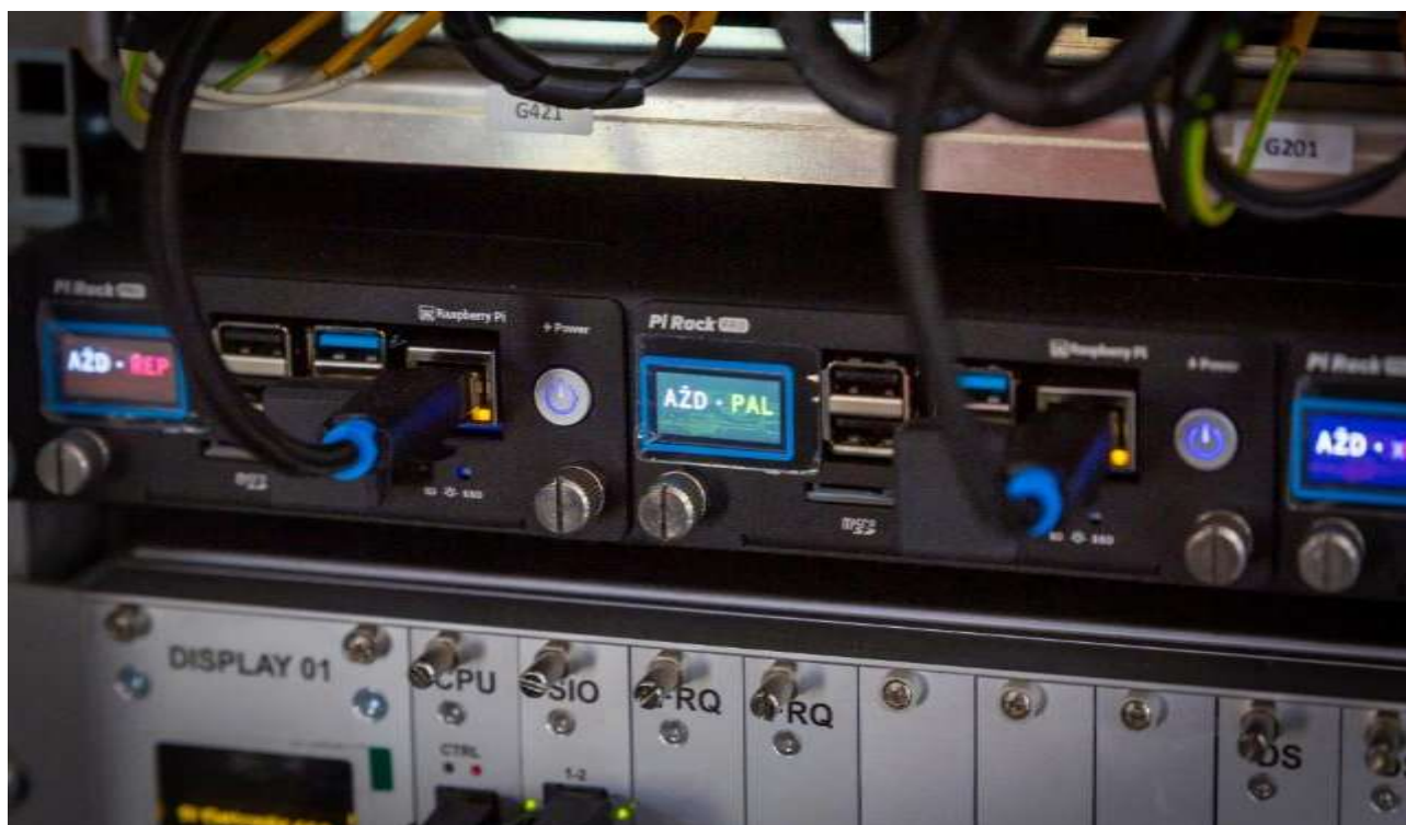
Figure 14: AZD Joint GoA3-4 computer - train installation
