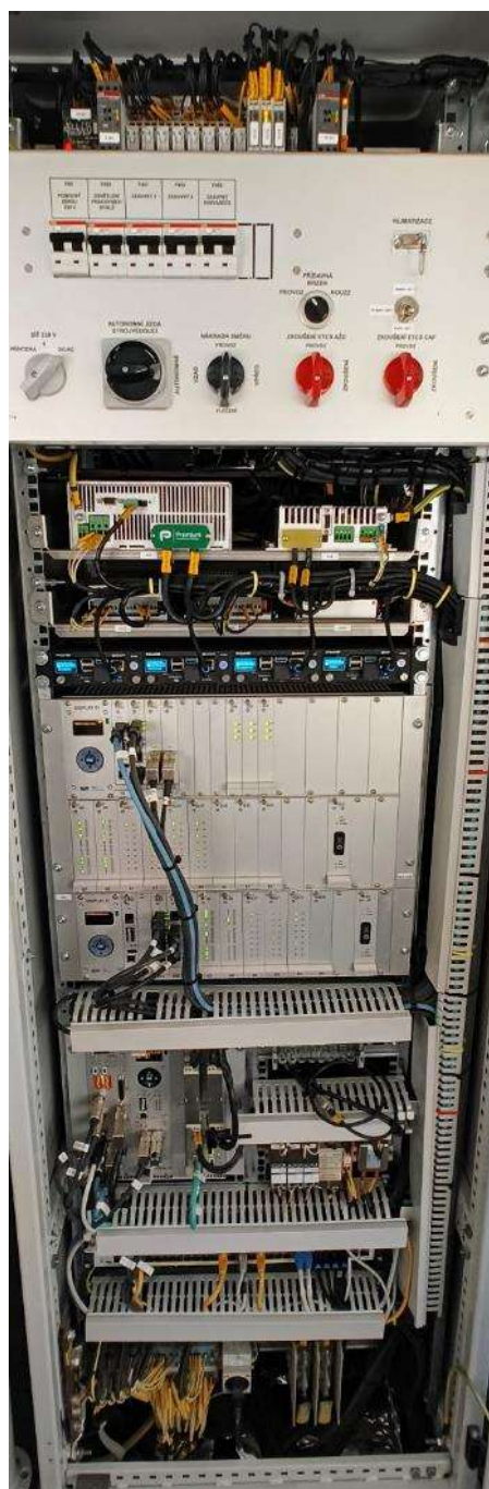
Figure 16: AZD R1 rack containing TCMS, ADM, anti-wheelslip, PAL and REP
