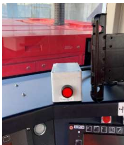
Figure 14 - Illuminated pushbutton on the remote control
