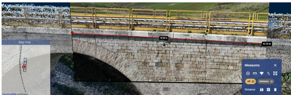
Figure 5-82: Linear measurement of a part of a bridge reconstructed with the point cloud
