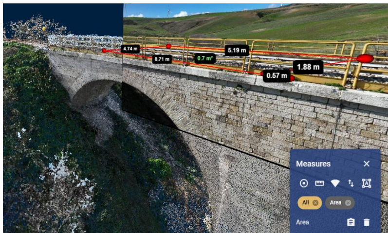
Figure 5-84: Area measurement of a part of the bridge reconstructed with the point cloud.
