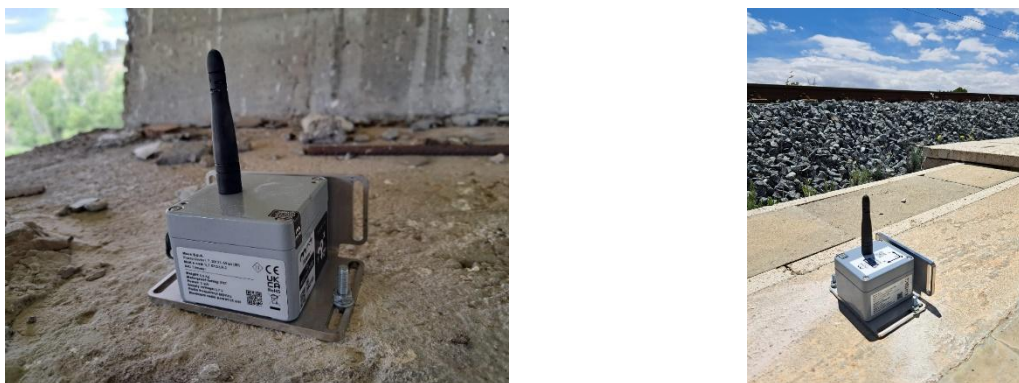
Figure 6-23: Tiltmeter installed on P11 and outside at the beginning of the bridge.
