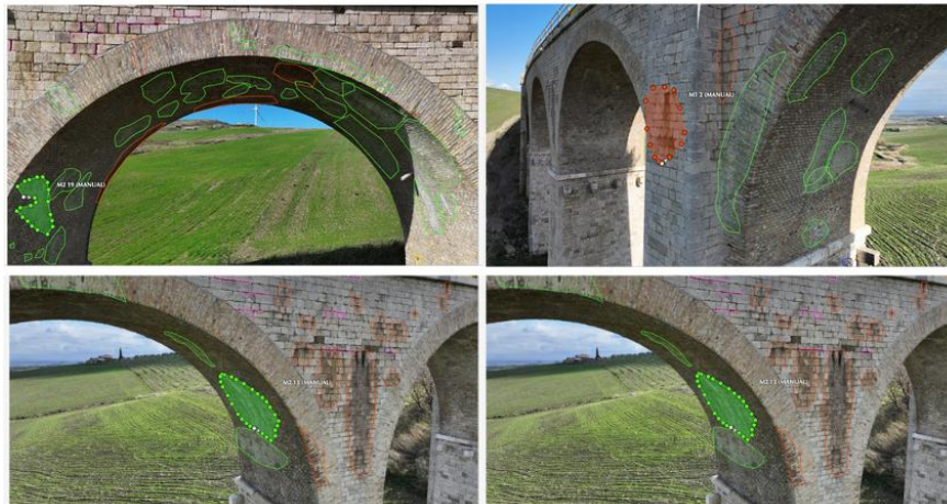
Figure 5-43: Examples of labelled defects in the Leonessa masonry bridge.
