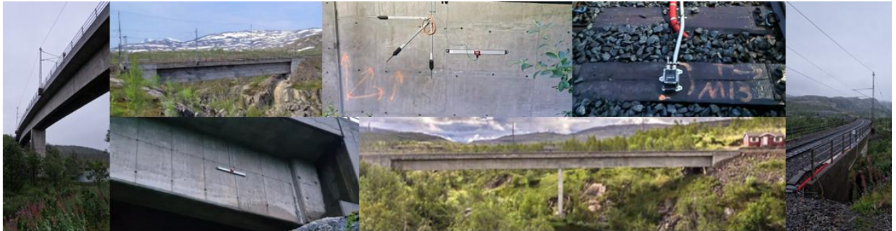
Søsterbekk bridges 1 (single span) and 2 (2-span) in Norway, with details about the accelerometers mounted on the sleepers in the transition zones and the inclinometers mounted along the bridge side.
