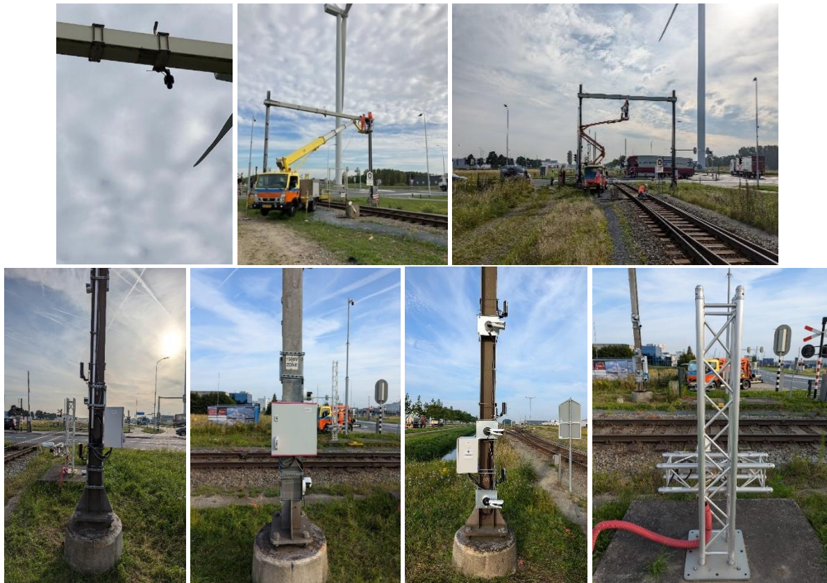
Figure 5.8 Photos of the IVG at Moerdijk
