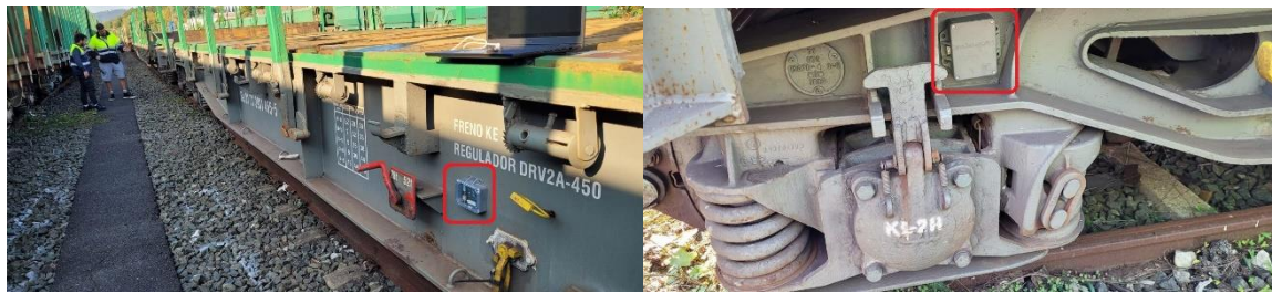
Figure 5.27. Location of a set of Wagon On-Board unit and sensors
