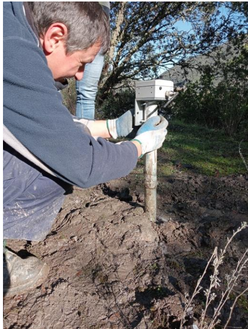
Image 2. Installation of clinometer on a mast embedded in the ground.
