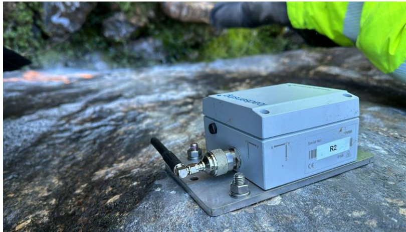
Image 7. Clinometer installed on a rock.
