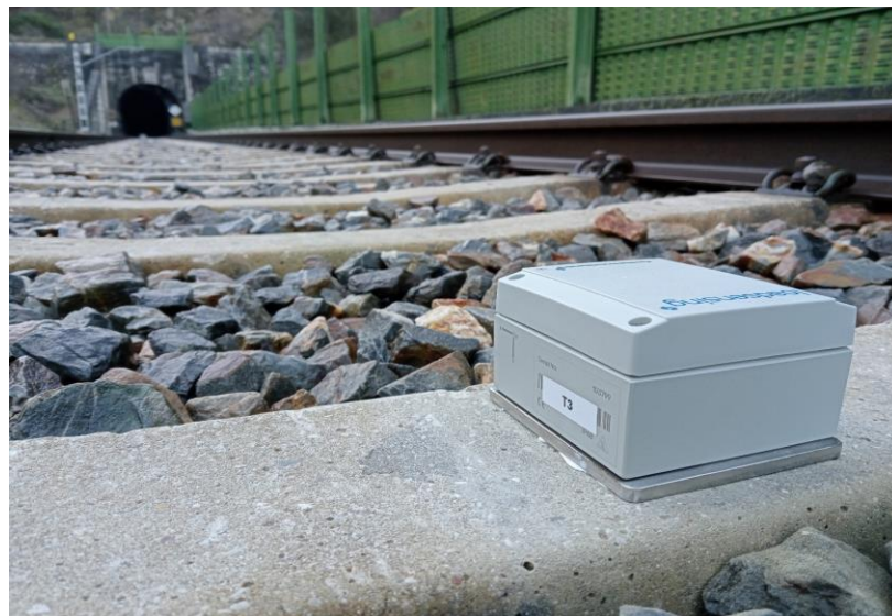
Image 8. Clinometer installed on sleeper.
