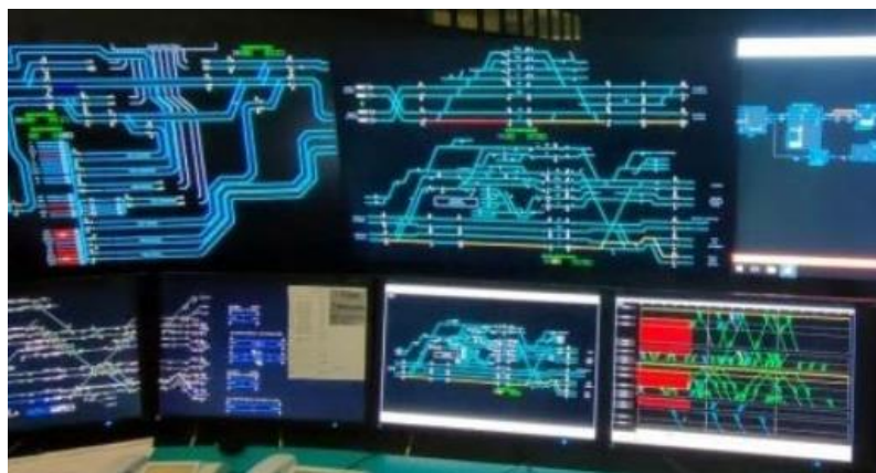
Figure 1: Example of Integrated Command and Control Center
