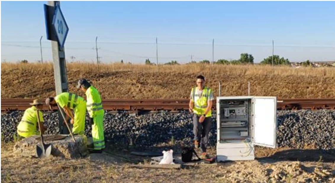
Rack in its final installation during its grounding
