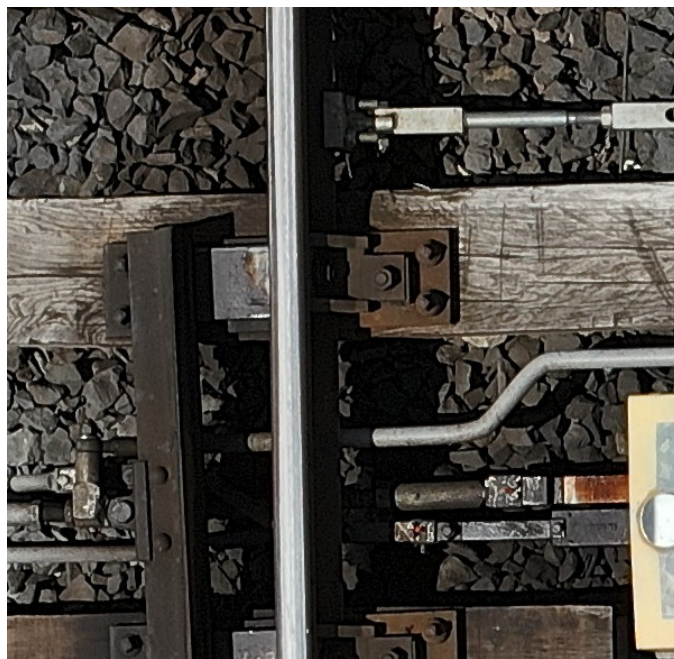
A detail of a switch captured by a drone with high resolution camera from 25 m altitude.
