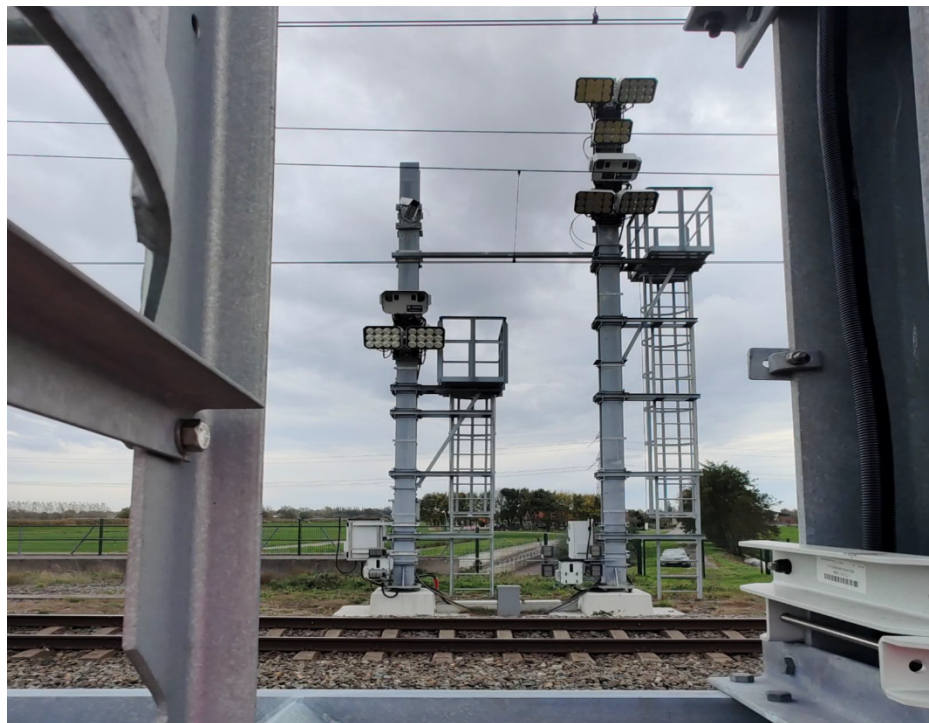
Photo: the pilot location with IVG's owned by NS and ProRail at Hogebrug
