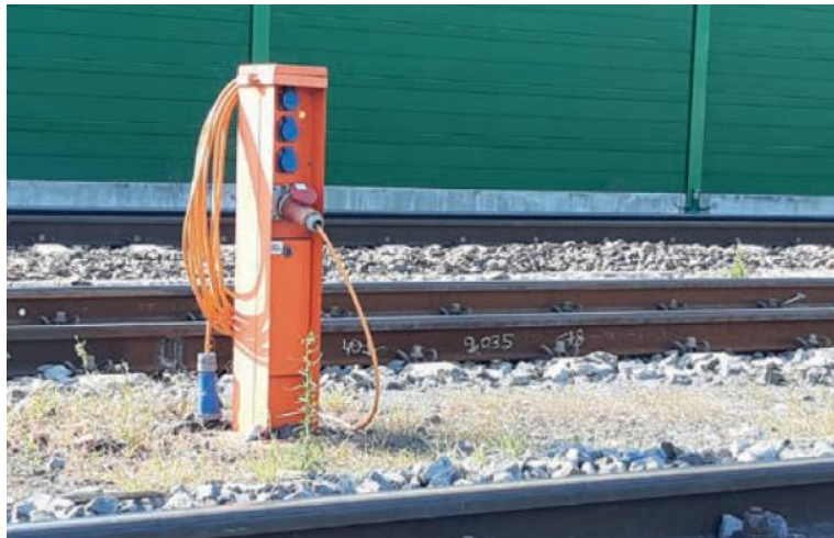
Figure 6: Parking energy supply for DMUs (32A, 22kW)
