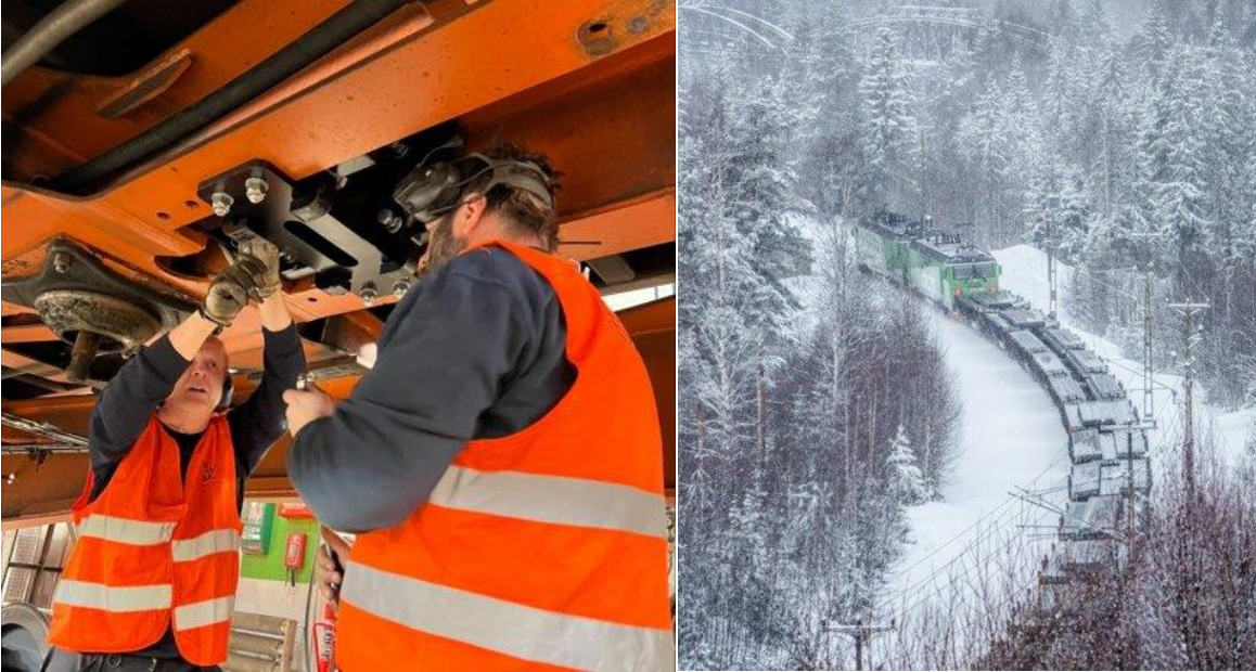
Installation and start of DAC commercial demo train in Sweden
